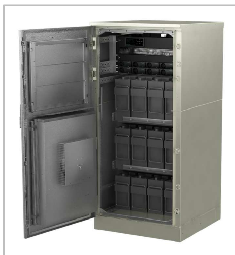
16kW Telecom system in outdoor cabinet
