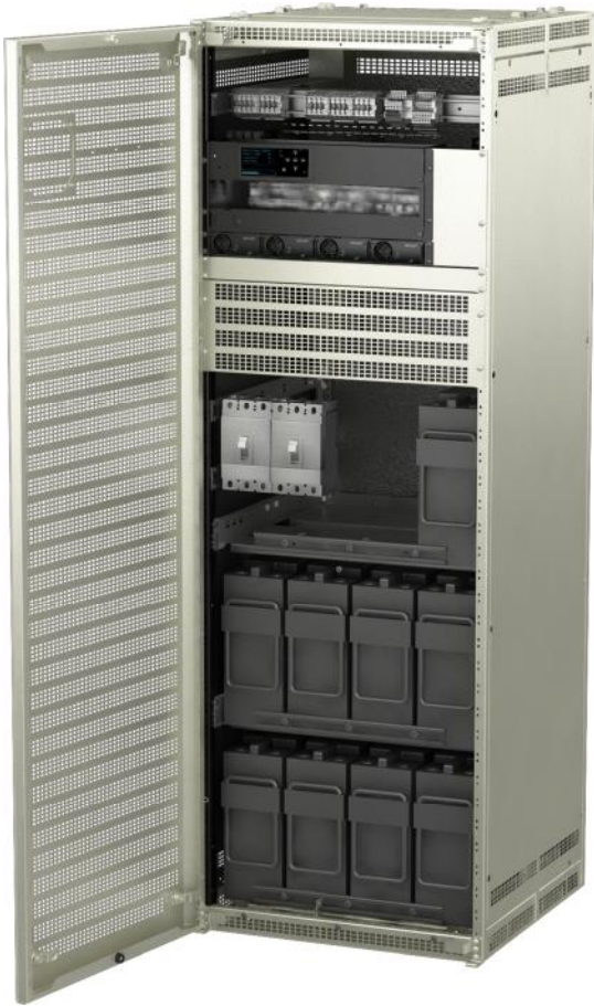
IBB SYSTEM IN FPC CABINET
